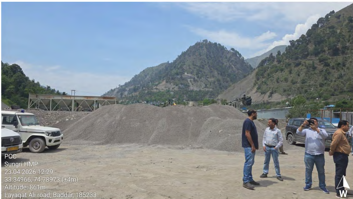
Pic-9: Wet Mix Macadam (WMM) Plant
