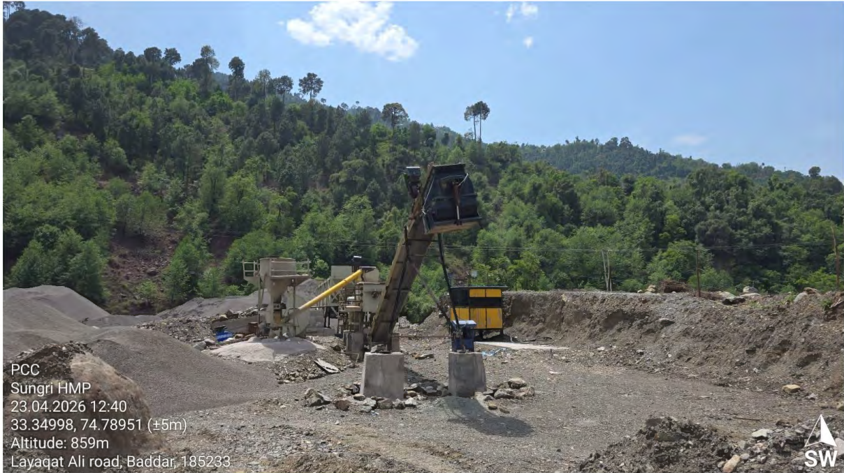
Pic-8: Wet Mix Macadam (WMM) Plant
